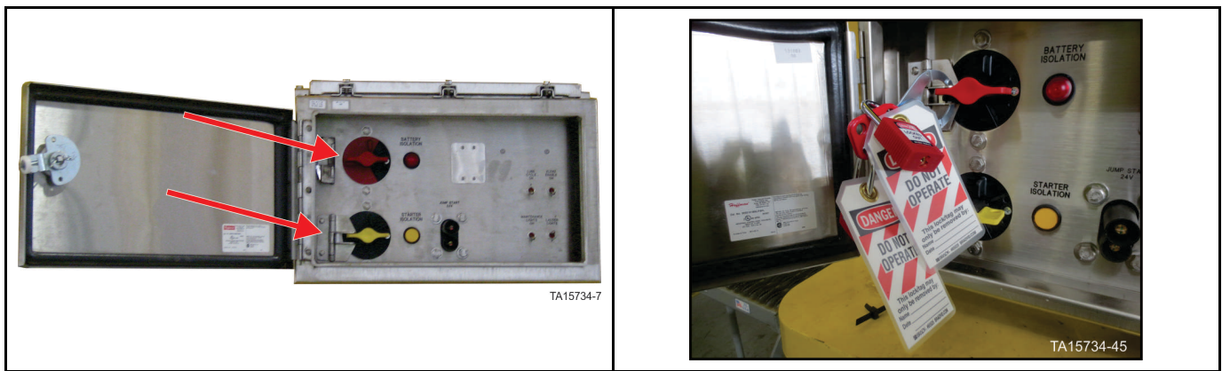
Figure 6: GEN 2 Battery Isolation Box – Battery isolation switch in OFF position with locks in place
