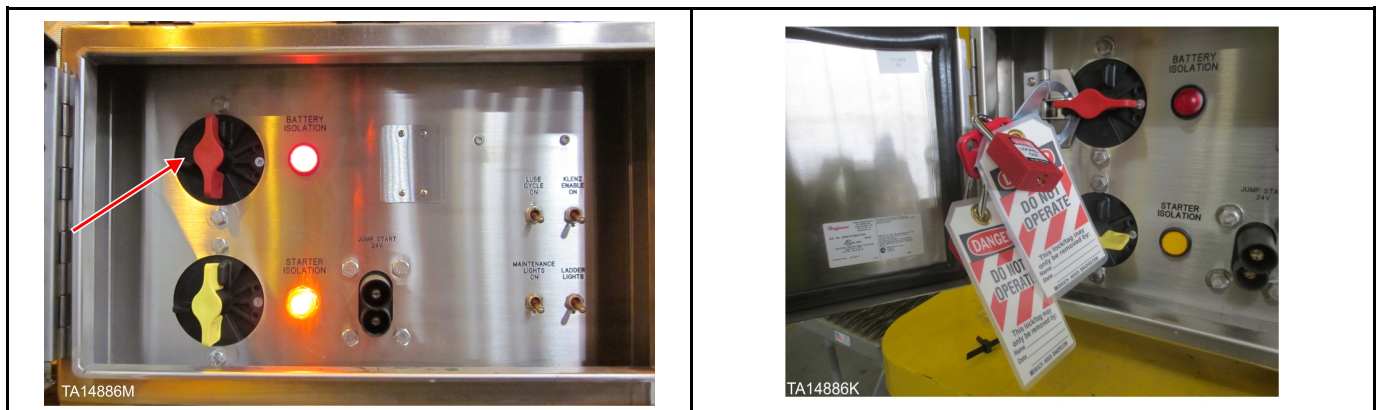
Isolate the battery and lockout the machine
