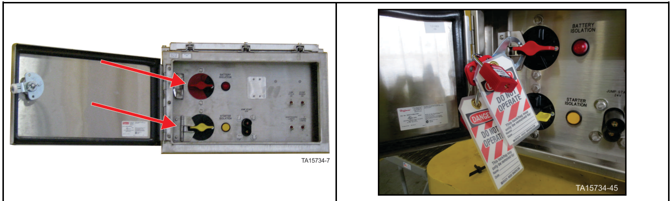
Figure 48: GEN 2 Battery Isolation Box – Battery isolation switch in OFF position with locks in place
