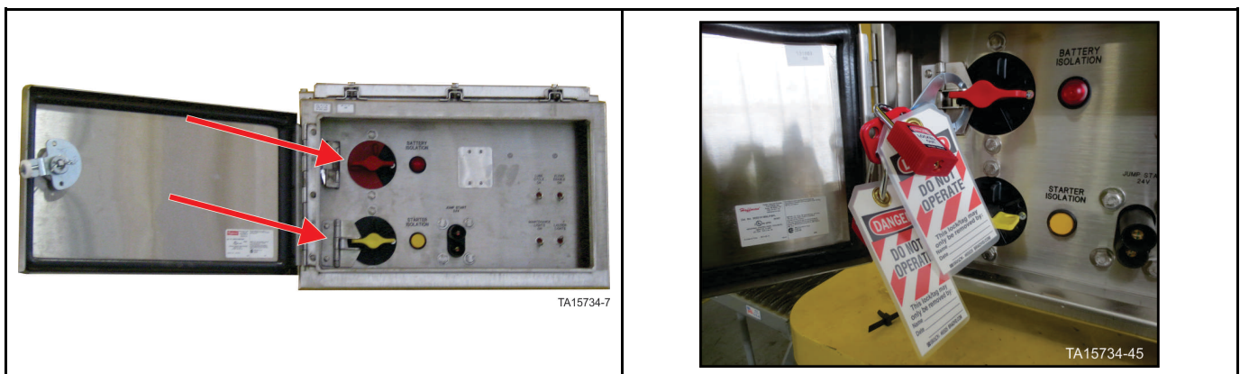
Figure 23: GEN 2 Battery Isolation Box – Battery isolation switch in OFF position with locks in place
